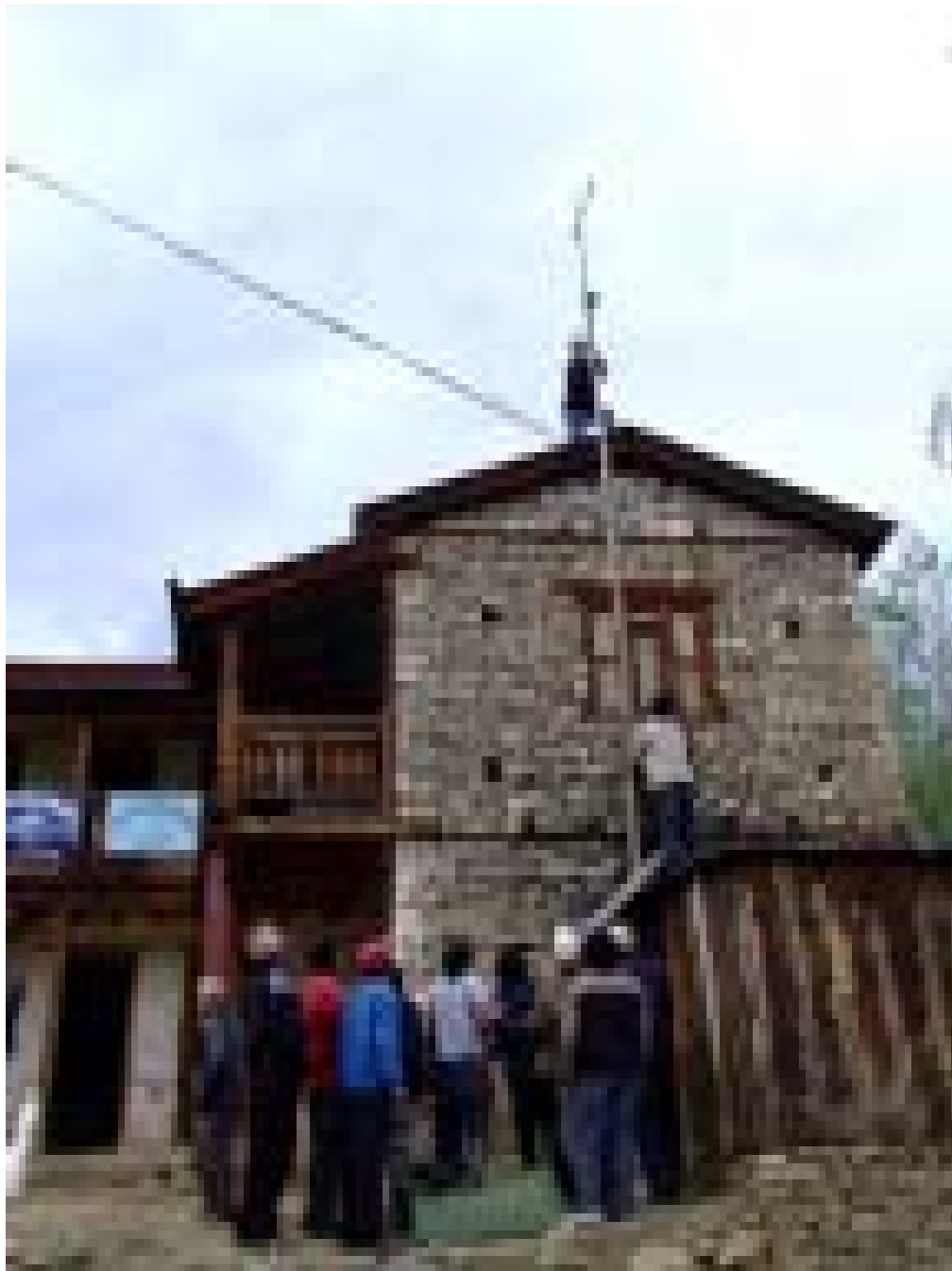
In Humla, the villagers set up the antenna on a tall rooftop. (MA)
